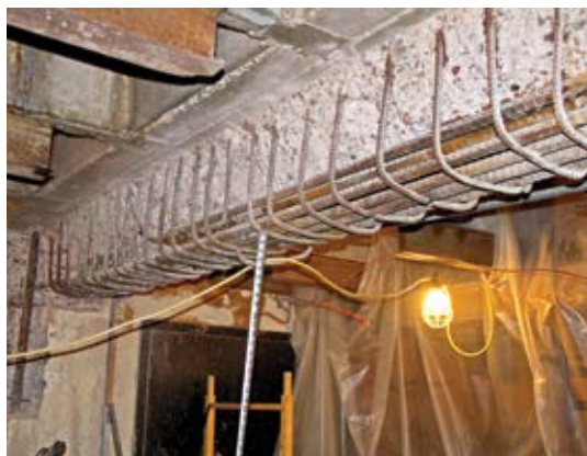
The start of concrete repairs to a beam. Note how ties on the right side are all broken from the expansive pressure of corrosion of longitudinal bars
