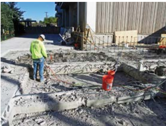
Complete removal and replacement of a portion of floor slab in front of building
